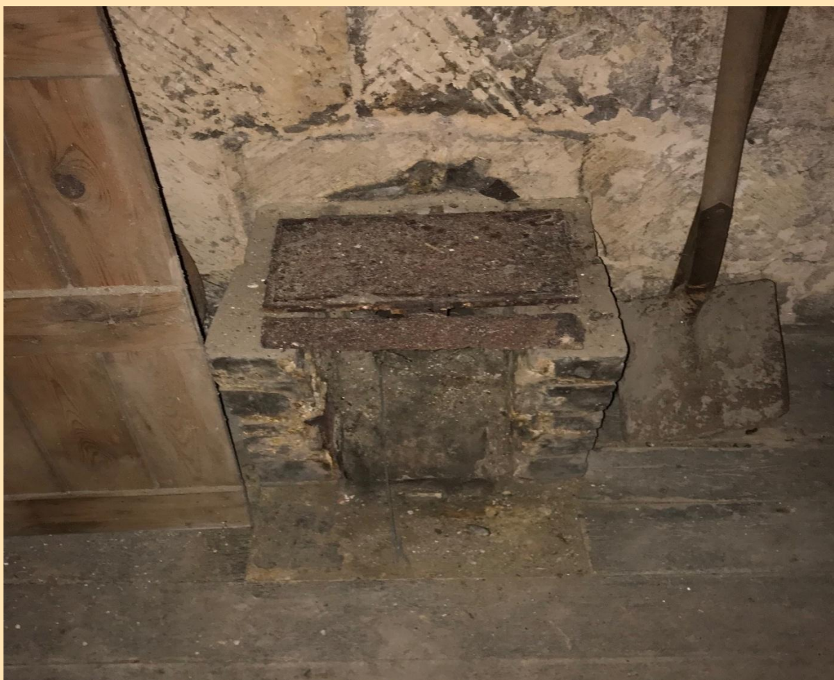
Inside the Clock Tower – A fire grate formerly used to keep the bell ringers warm
